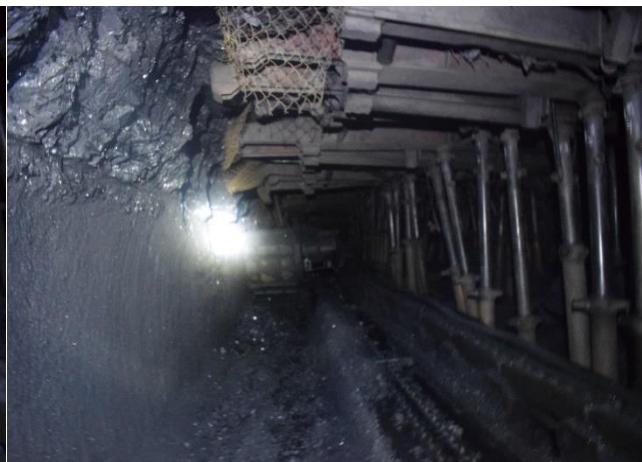
Figure 4. Hydraulic supports are not close to coalface at longwall face I-6-2.
